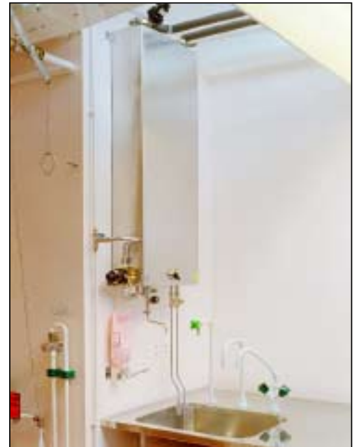
Fig 2. Installation of a Pharma-X module as a point of use cooler at AstraZeneca, Södertälje, Sweden.
